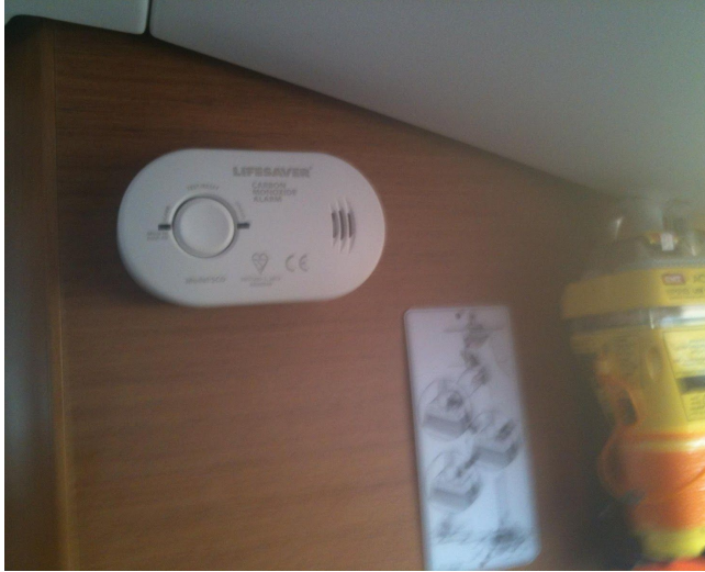
CO Alarm Main Cabin
